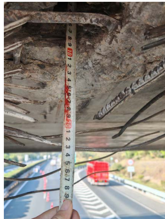
图3-6: 3-1空心板梁底板空洞孔洞
