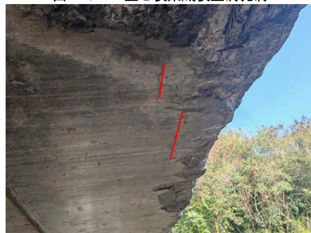
图3-8: 3-1空心板梁底板纵向裂缝
