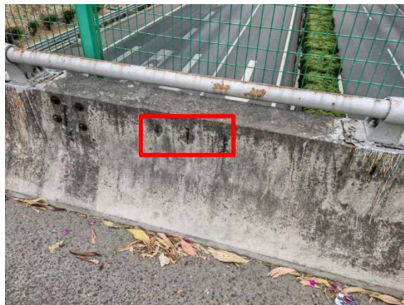
图3-2: HL-R-1护栏内侧露筋
