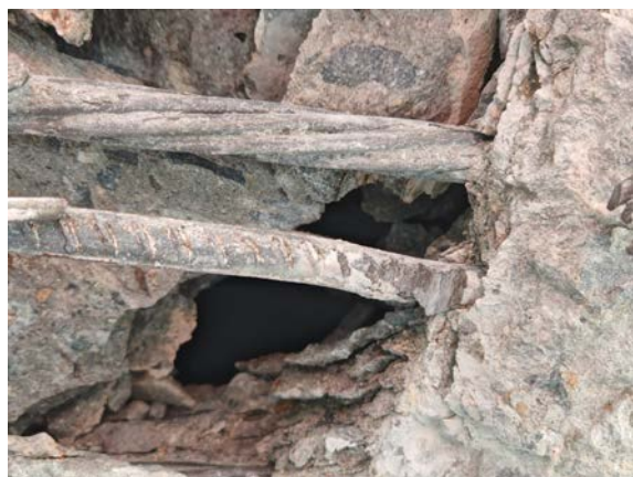
图3-5: 3-1空心板梁底板空洞孔洞
